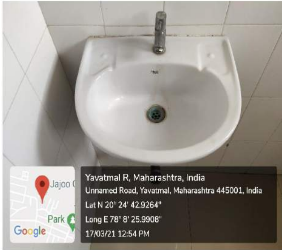
Taps to be replaced by Faucets
