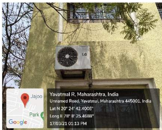
AC Condenser in shade
