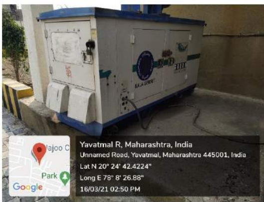
Diesel Generator in college
