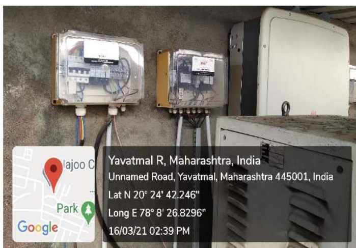
Solar PV System installed in college
