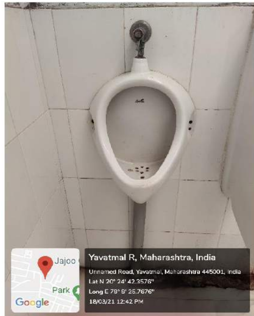
Flush to be replaced by Push Buttons
