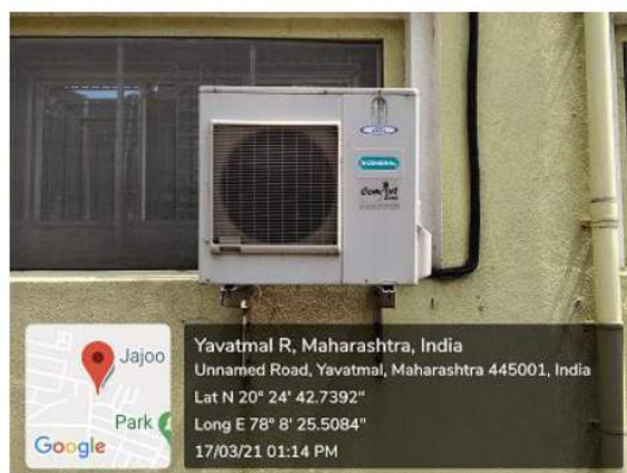
AC Condenser directly exposed to sunlight
