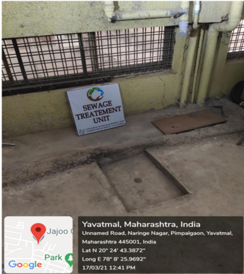
Sewage Disposal System in college building
