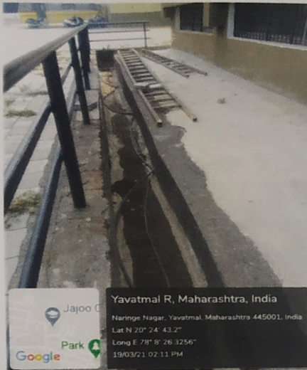
Drainage System Connected to Water Harvesting Pit
