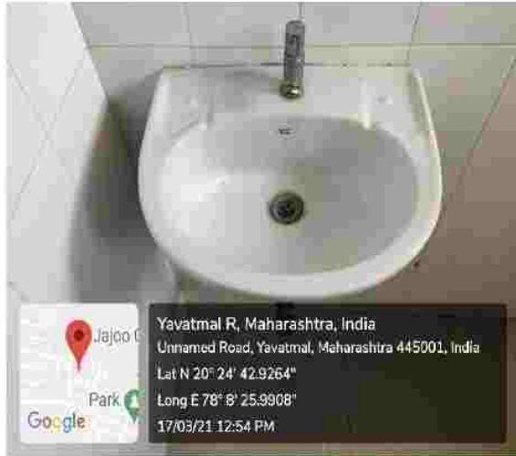
Taps to be replaced by Faucets
