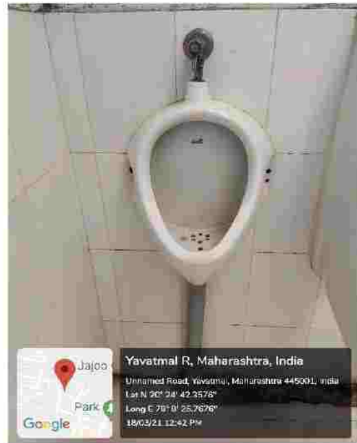
Flush to be replaced by Push Buttons
