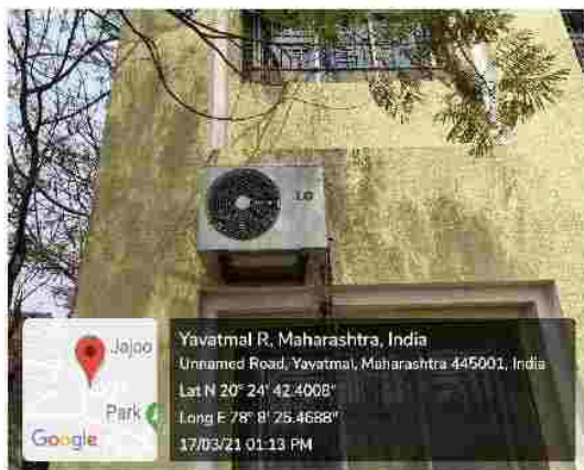
AC Condenser in shade
