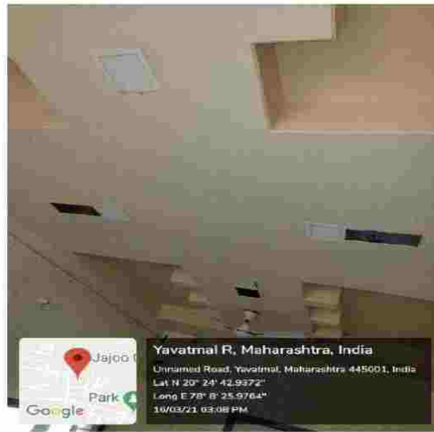
Use of false ceiling to reduce air-conditioned volume and reducing AC load
