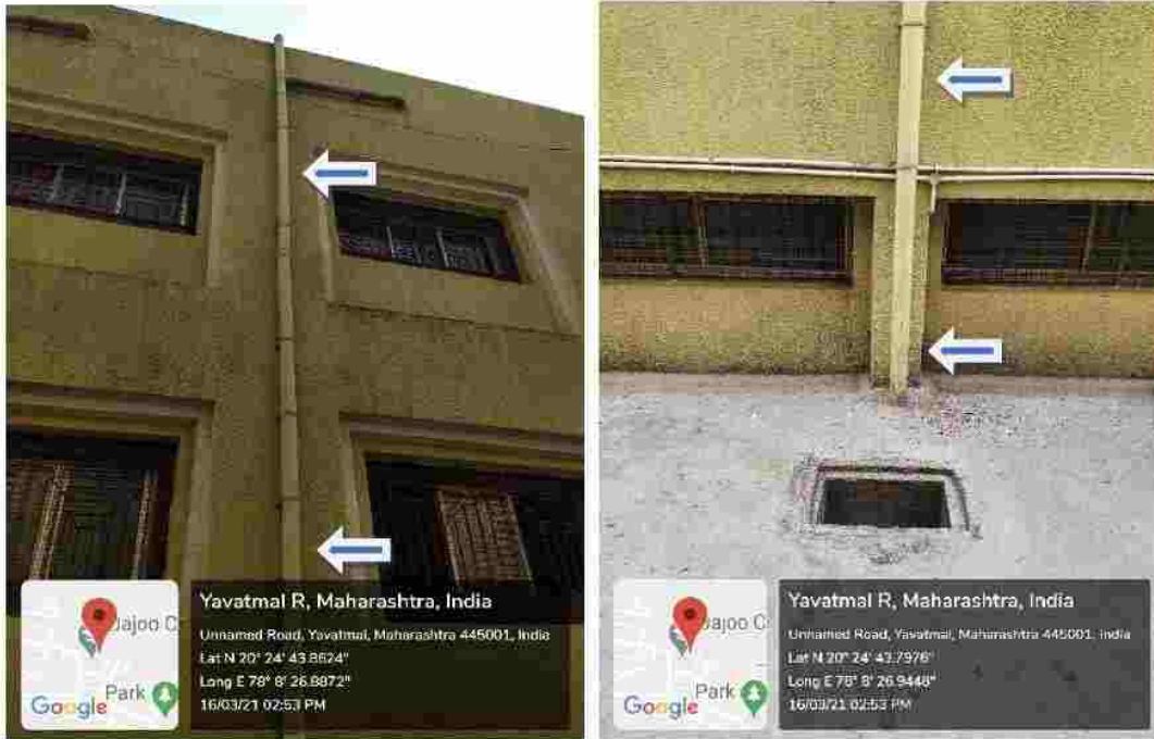
Pipeline of Water Harvesting System
