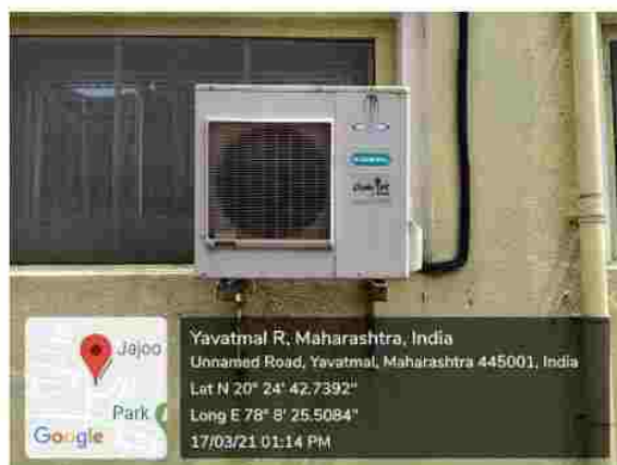
AC Condenser directly exposed to sunlight
