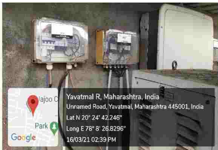
Solar PV System installed in college
