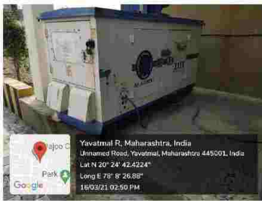
Diesel Generator in college
